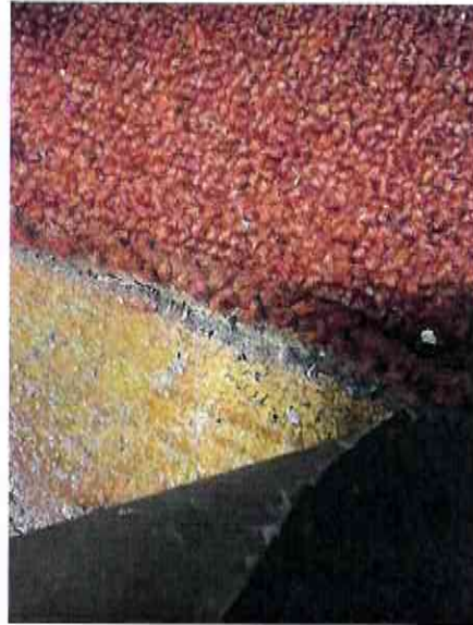
Floor Area under carpet – No Floor Tile
