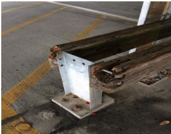
Photo #M13 – Rotted Timber Guardrail
