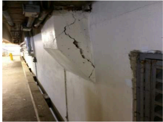
Photo #U8- Crack at Column Corbel
