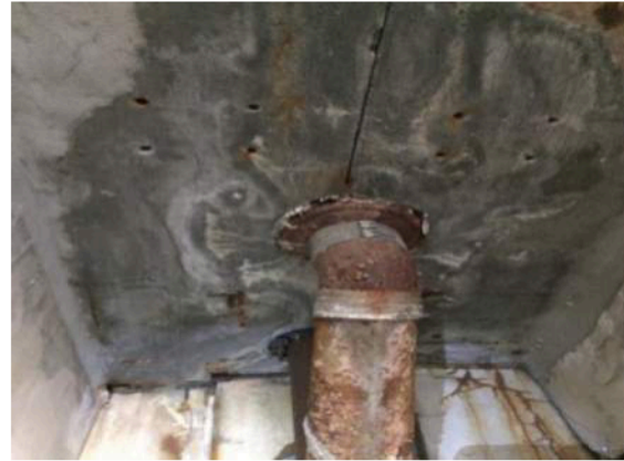
Photo #U14- Rusted Floor Drain and Pipes
