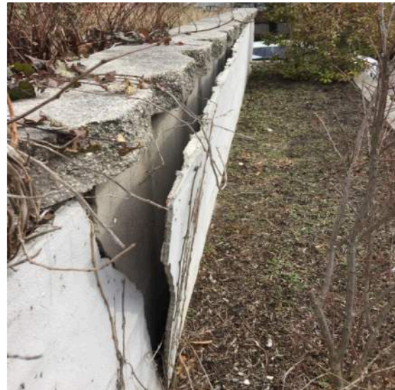
Photo #R4- Failing Sections in the Upper Wall Stucco
