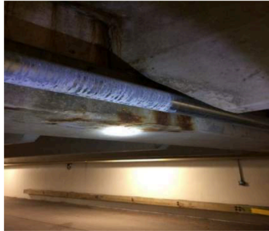
Photo #M8- Crack at “T” Girder and Beam
