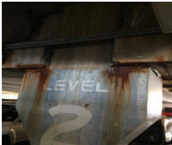
Photo #U5 – Spall at Col./Corbel
