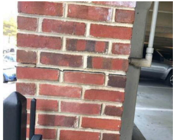
Photo #U16 – Joint Crack in Exterior Brick
