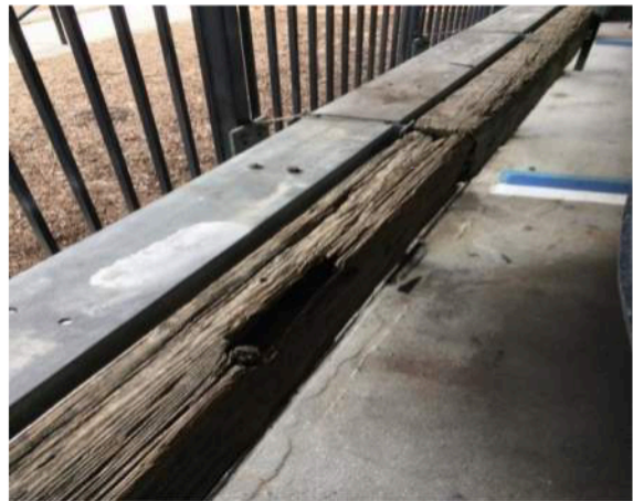
Photo #U12- Rotted Timber Guardrail
