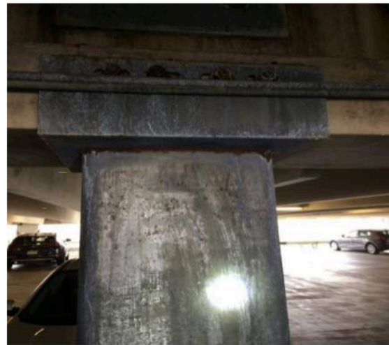
Photo #M16 – Minor Rust at New Steel
