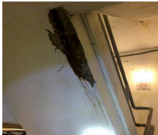
Photo #M6- Spall at Stairs
