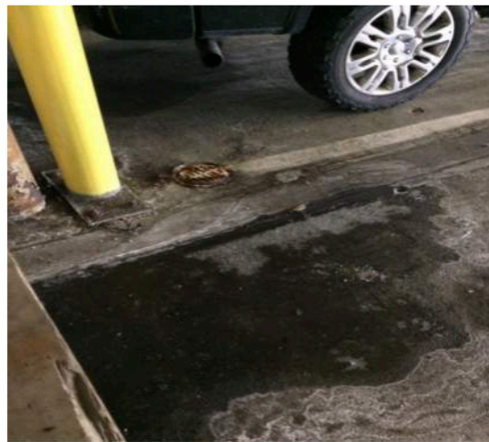
Photo #M10- Water Ponding
