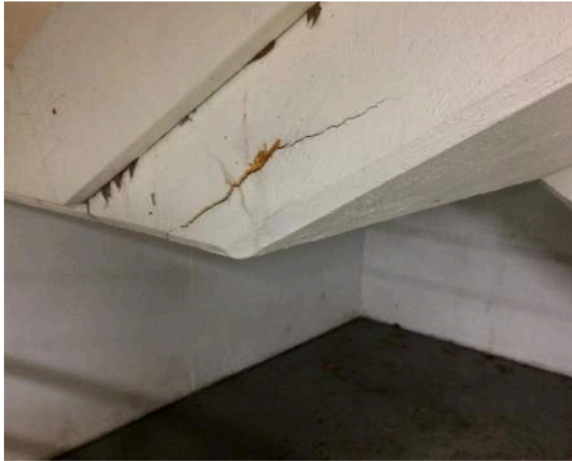
Photo #M7 – Crack at Stair
