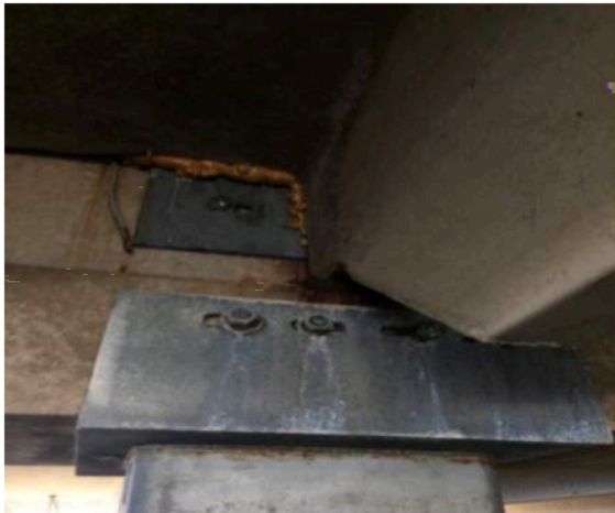
Photo #U15 – Minor Rust at New Steel
