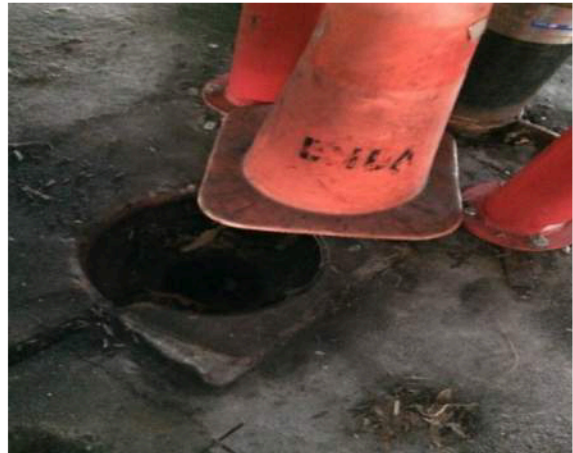
Photo #U10 – Clogged Drain Pipes
