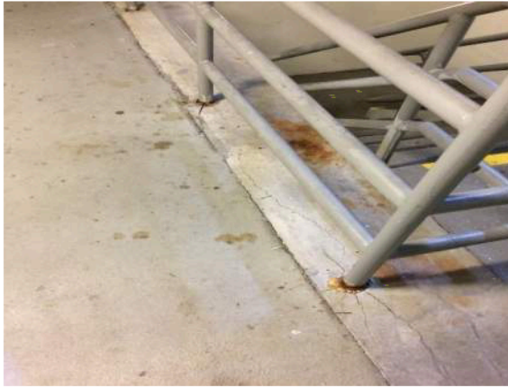
Photo #U7 – Crack at Stair Railing
