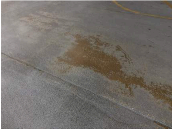
Photo #U13 – Worn Down Traffic Surface
