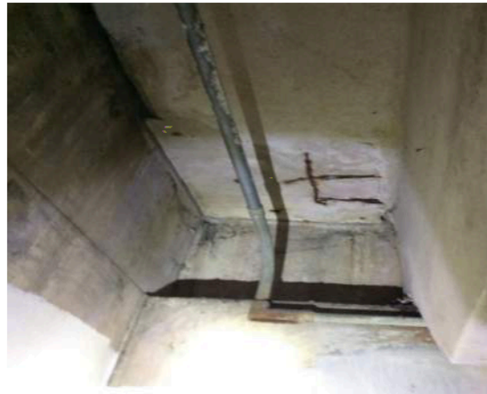
Photo #M4- Spall in “T” Beam
