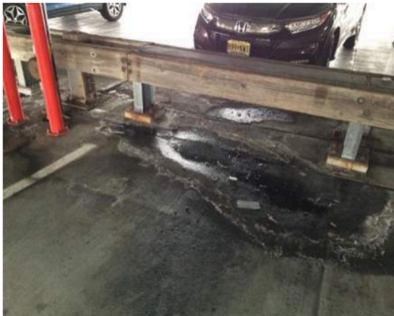
Photo #U9 – Water Ponding
