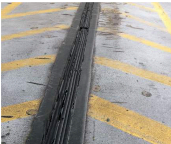
Photo #U17 – Deteriorated Expansion Joint
