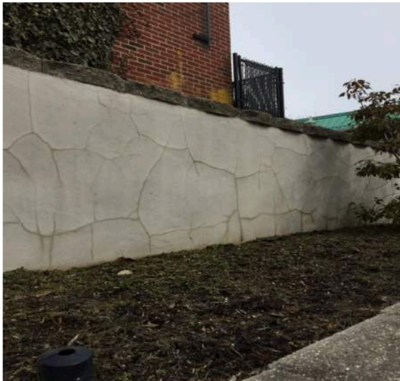
Photo #R3- Cracking in the Upper Wall Stucco
