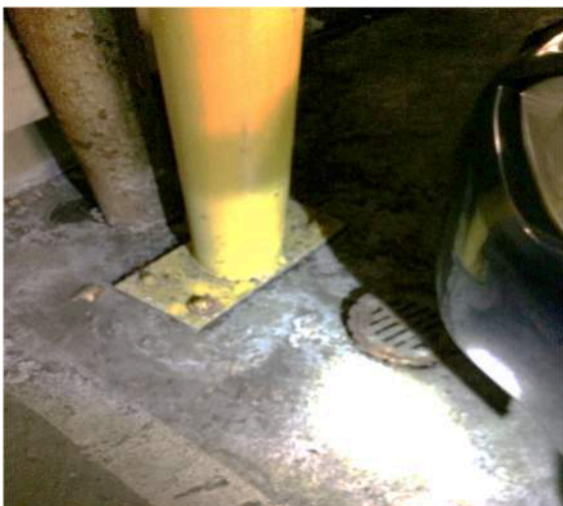
Photo #M11 – Clogged Drain Pipes
