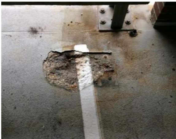
Photo #U11 – Bolts from Removed lights
