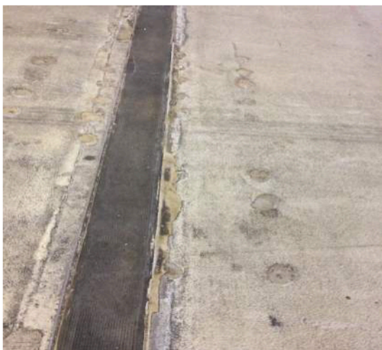
Photo #M15- Deteriorated Expansion Joint
