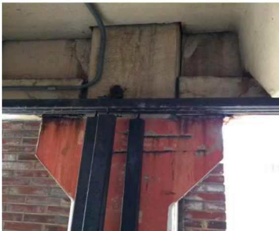
Photo #M5 – Spall at Col./Corbel
