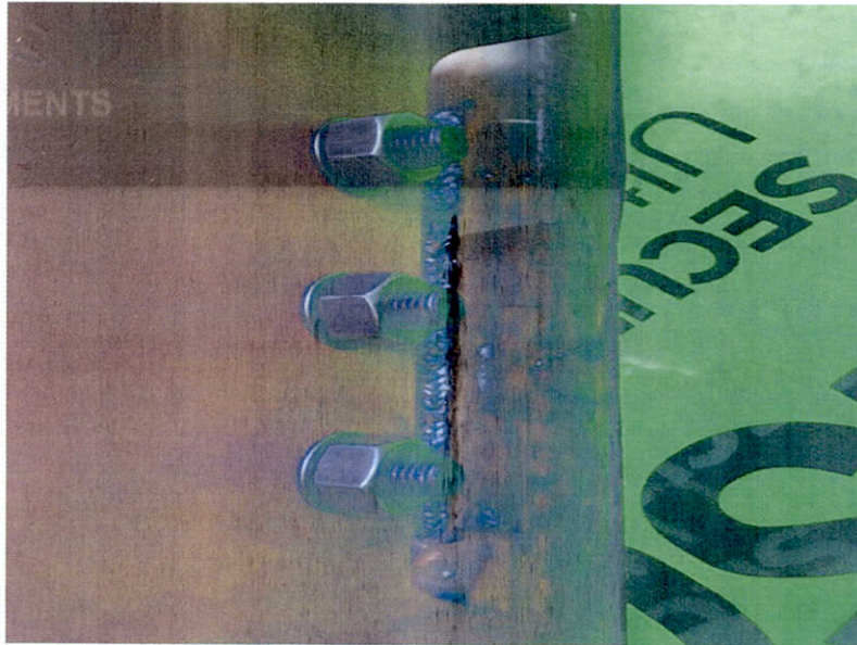
Attachment No. 3 Sheared Bolts, 0.25-inch Fillet Weld New Framing To Existing Structure
