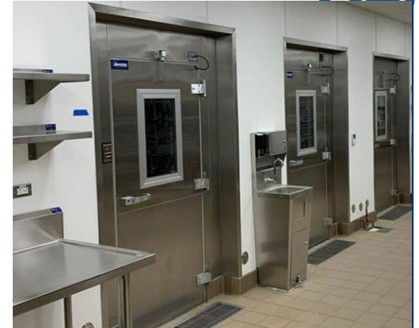
WALK-IN REFRIGERATOR & FREEZER CONTROLS
