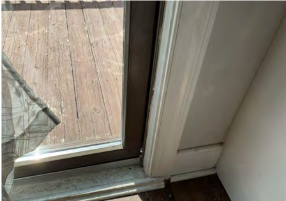
42030, Doors not sealing
