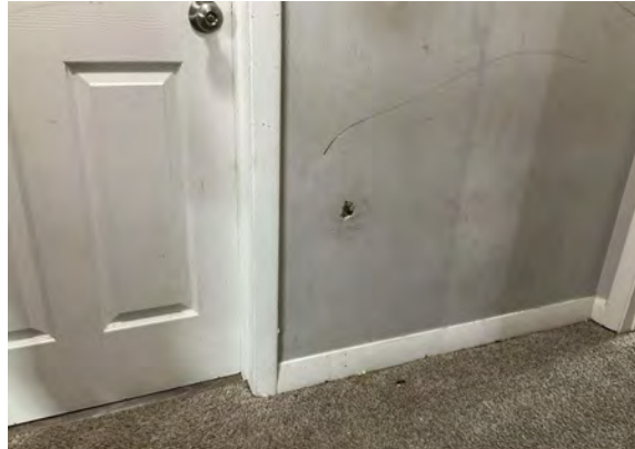
42044, Holes on the walls
