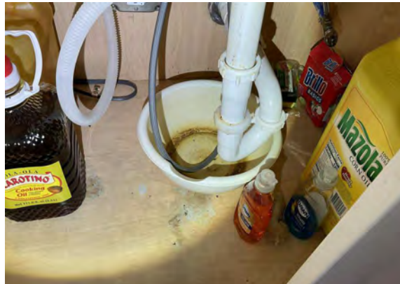
42017, Leak kitchen sink
