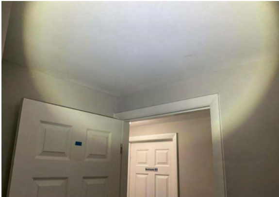
42024, Alarms missing throughout
