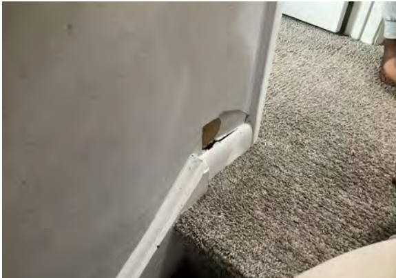
42045, Holes on the walls
