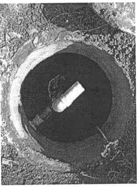
Pump tank access.
