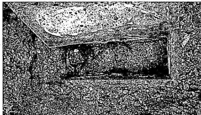
Deteriorated & Sludge Fouled D-Box
