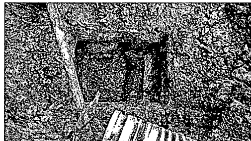
Southern Septic Tank Outlet Opening (Note Elevated Liquid Level & Eroded Outlet Baffle)
