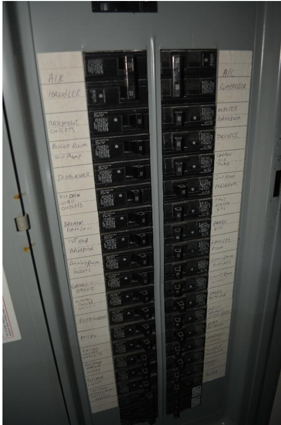
Breakers 11,12,24,28,32 in the tripped position
