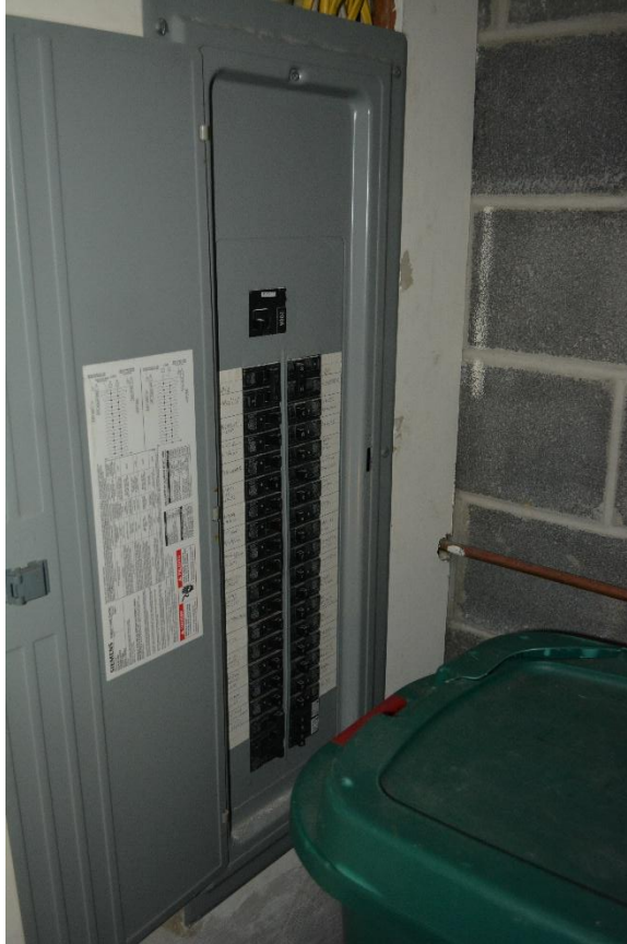
Siemens electrical panel
