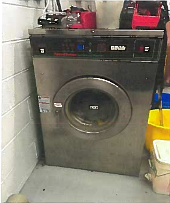
VINCENT FIRE COMPANY TURNOUT GEAR WASHER
