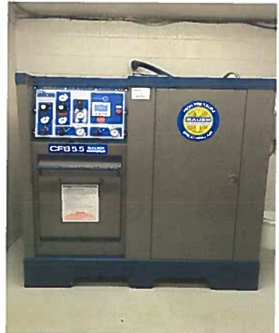
VINCENT FIRE COMPANY SCBA AIR CYLINDER FILL STATION
