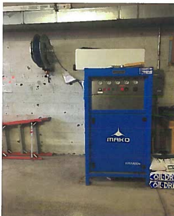
HAMPTON LAKES FIRE COMPANY SCBA AIR COMPRESSOR FOR CASCADE SYSTEM
