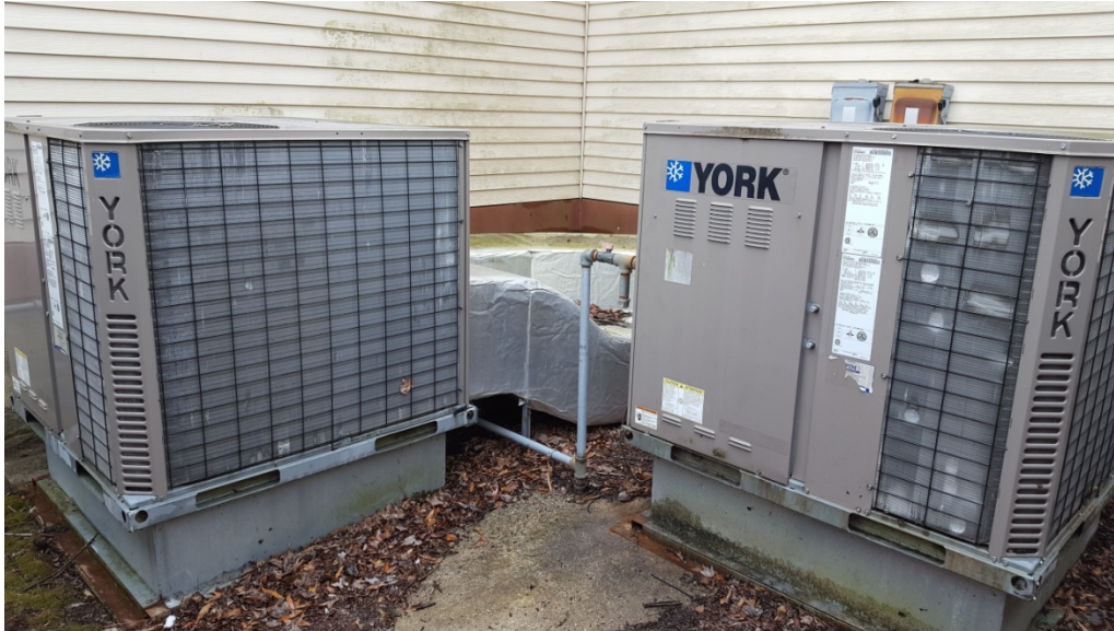
View of heating equipment at Community Center
