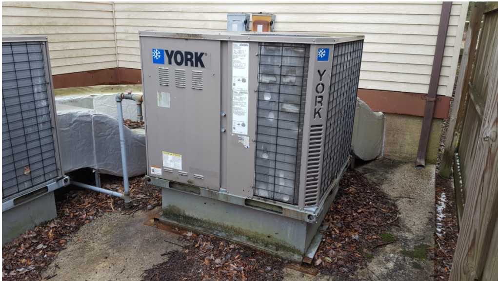
View of heating equipment at Community Center
