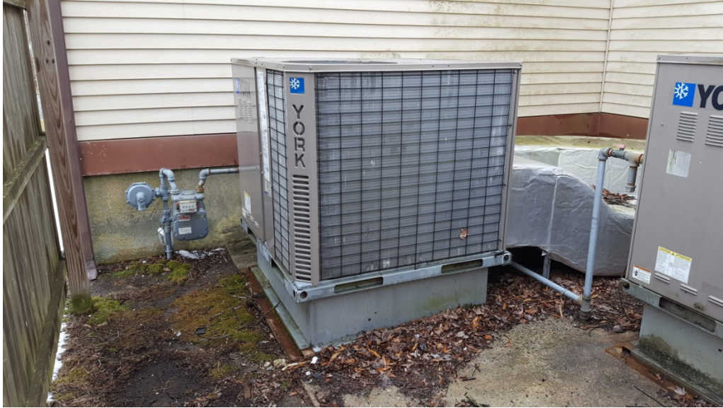
View of heating equipment at Community Center
