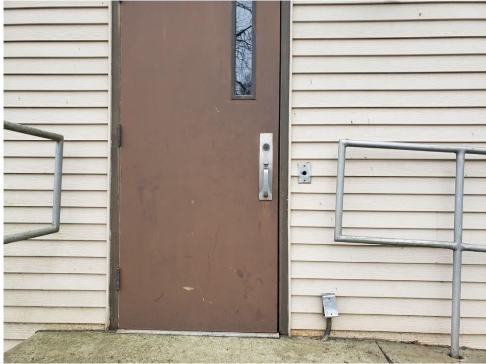
Existing concrete ramp entrance door with non-compliant hardware and opener.
