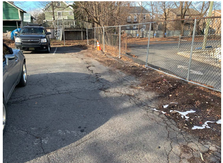
Figure 2: Deteriorated pavement in northwest corner of Lot 28.
