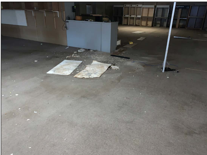
Figure 9: Debris from fallen, water damaged ceiling panels.
