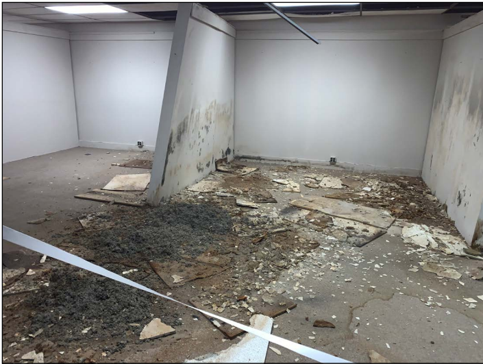
Figure 7: Debris and water damage from collapsed roof/ceiling.
