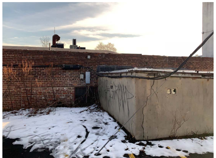
Figure 18: Deteriorated addition at rear of building.
