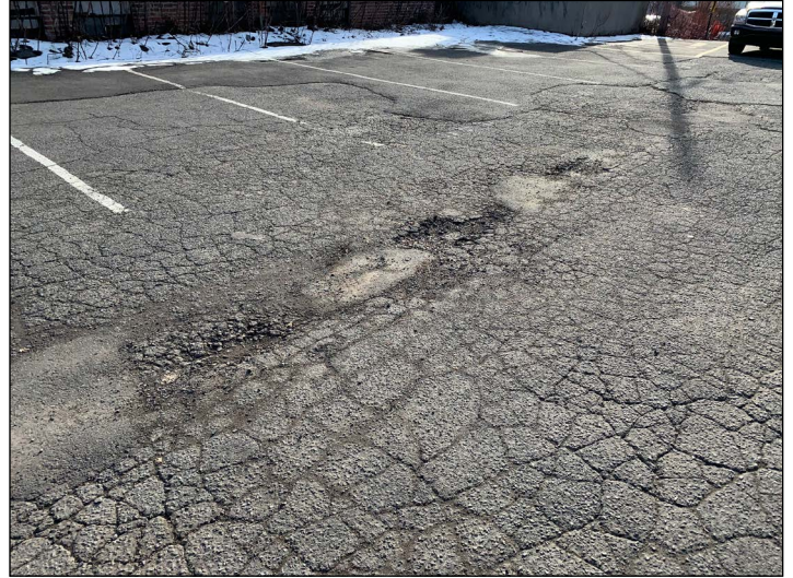
Figure 6: Deteriorated pavement in access aisle on Lot 28
