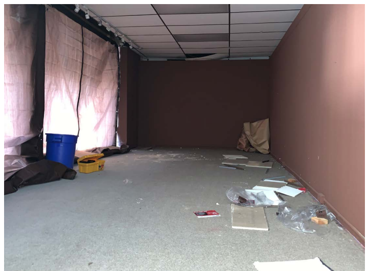
Figure 12: Vacant interior area with garbage accumulating.
