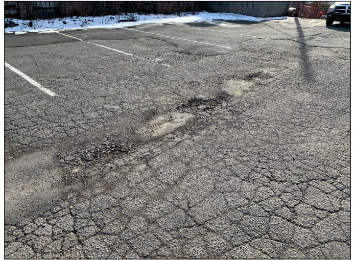
Figure 6: Deteriorated pavement in access aisle on Lot 28
