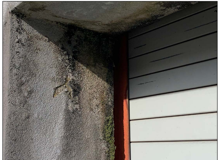
Figure 16: Wall damage near loading door.
