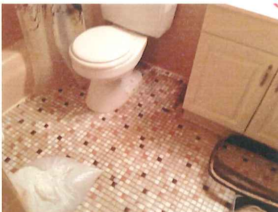
Unit 50- Affected Bathroom
