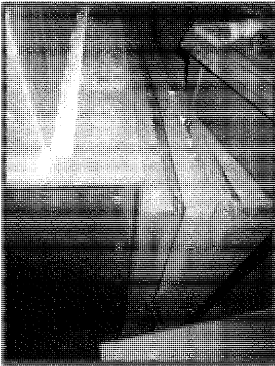
HVAC Duct Joint Vibration Cloth Determined to be ACM during previous inspection activities per County of Manmouth Records
