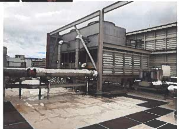
Existing 2-cell cooling tower (to be replaced)
