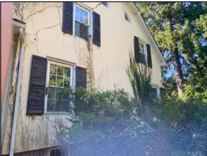
Figure 41: View of vacant Lutkins house side facade with overgrowth.
