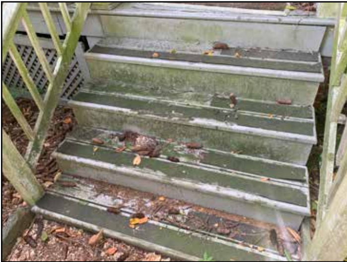
Figure 43: View of vacant Lutkins house front steps in poor condition.
