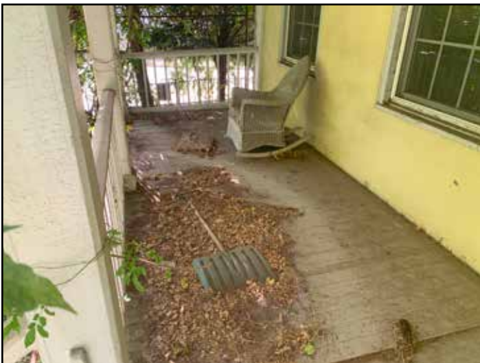
Figure 47: View of vacant Lutkins house rear porch in poor condition.
