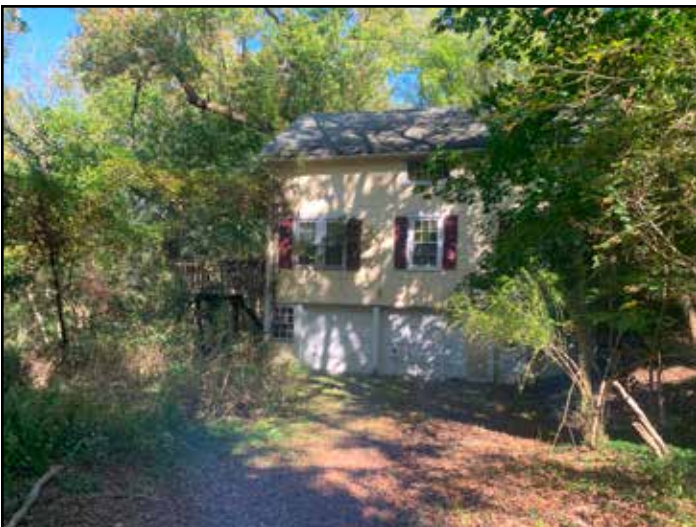
Figure 23: Vacant Mill House side facade with overgrowth.
