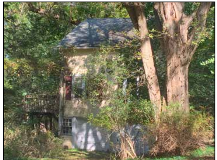
Figure 24: Vacant Mill House side facade with overgrowth.
