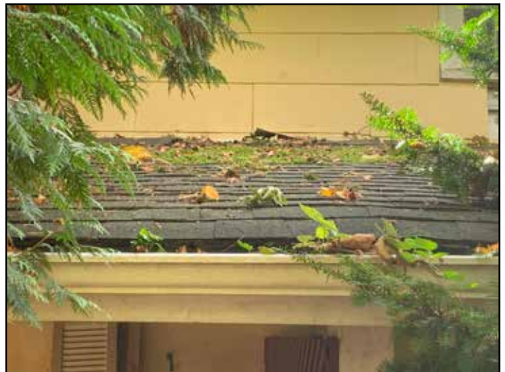
Figure 28: Vacant Mill House with moss and buckling on the roof.
