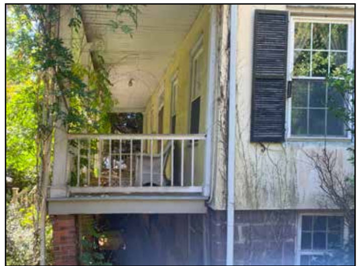
Figure 46: View of vacant Lutkins house rear porch in poor condition with column falling.
