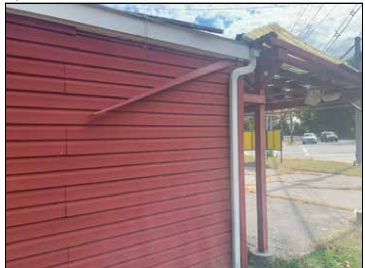
Figure 10: Vacant former garden center commercial building with siding falling and trellis damage facing the corner.
