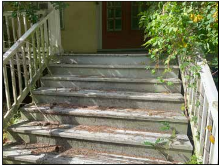
Figure 38: View of vacant Lutkins house rear porch steps in poor condition.
