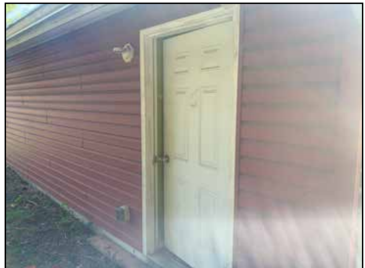
Figure 12: View of the rear with partially broken in back door.
