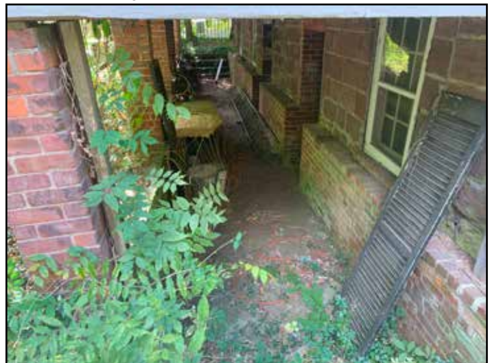
Figure 48: View of vacant Lutkins house rear walkout area from the basement in poor condition.
