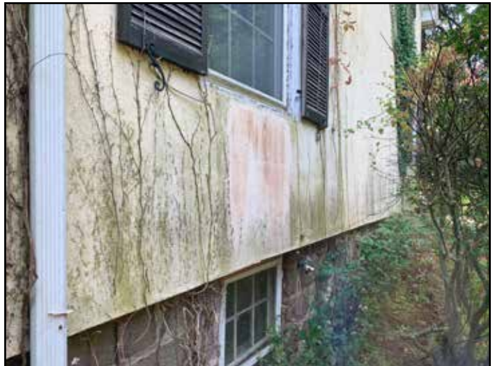
Figure 42: View of vacant Lutkins house side facade with overgrowth.
