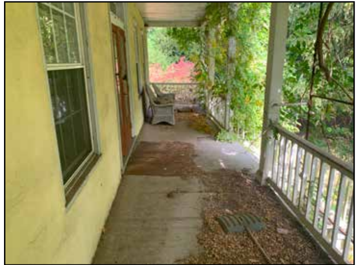
Figure 44: View of vacant Lutkins house rear porch in poor condition.
