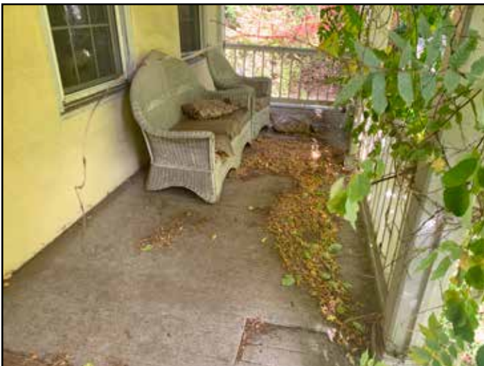
Figure 45: View of vacant Lutkins house rear porch in poor condition.
