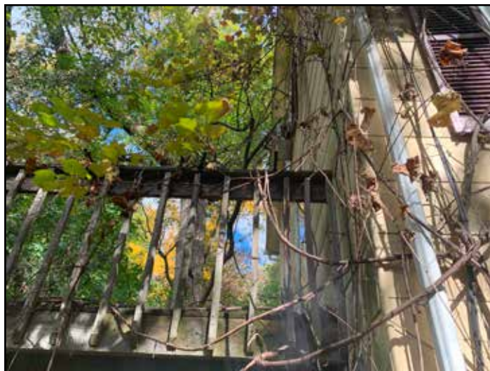
Figure 32: Vacant Mill House rear porch deteriorating with overgrowth.
