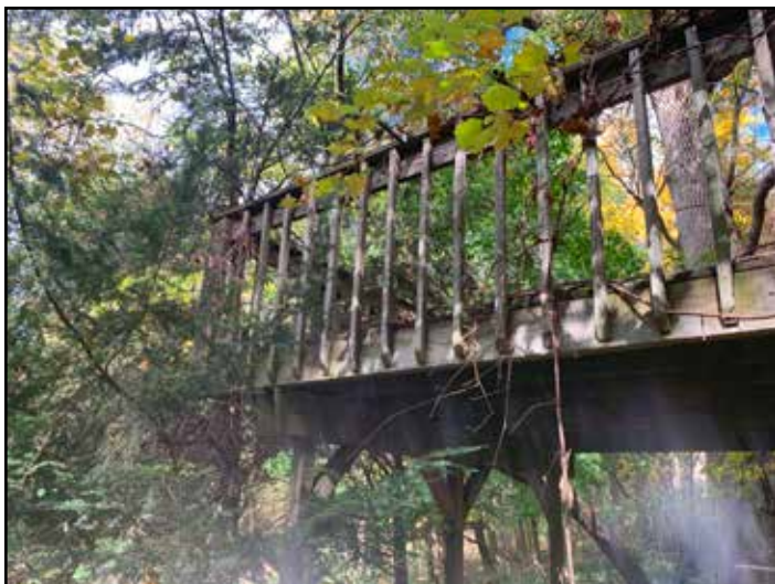
Figure 31: Vacant Mill House rear porch deteriorating with overgrowth.
